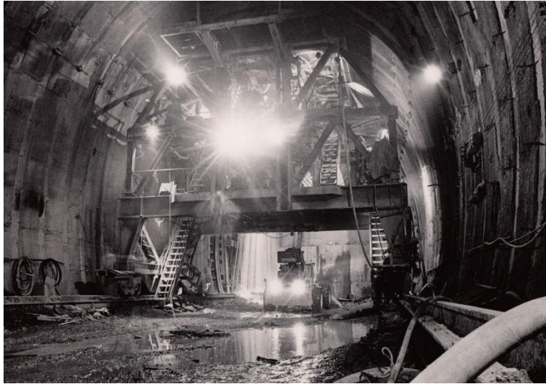
Inside the bore for the Eisenhower tunnel in 1971. Loyd Files Research Library photo
